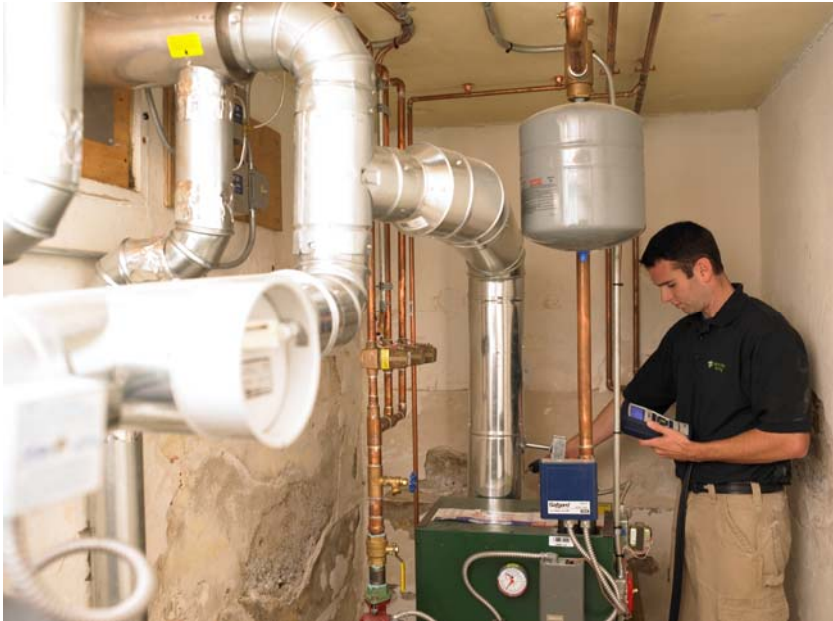
Technician checking carbon dioxide level and efficiency of oil furnace
