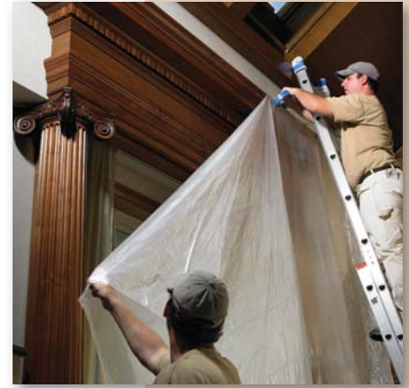
Site protection is necessary to avoid paint dust from penetrating the rest of the house.
